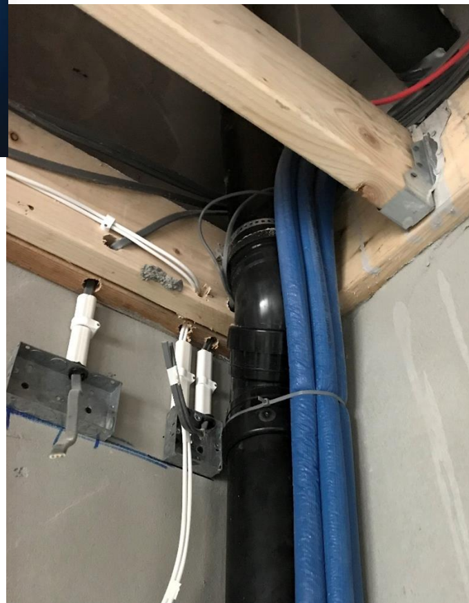
Bunched service penetrations fit tightly to corners which cannot be individually taped or sealed
