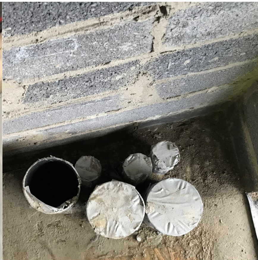
Bunched service penetrations in a floor which cannot be sealed individually
